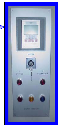
FRONT PANEL FEATURING KWH METER
